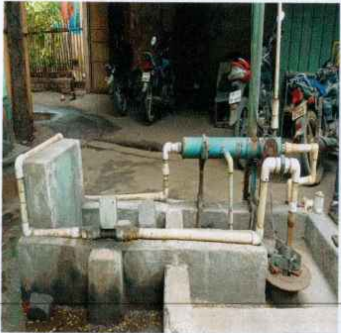
Digital Water Meter in Borewell at gate No. 3
